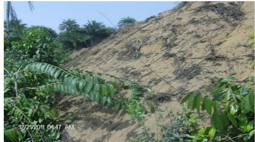
Deposit of excavated earth spread for reclaiming mashed eroded land along shore of lagoon.
